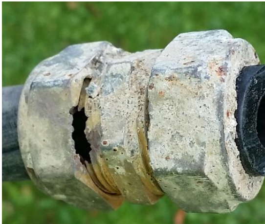
Leak - Poor Quality Fittings
