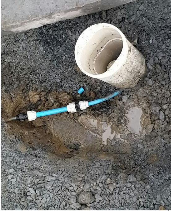
Leak on existing DCC Boundary Box
